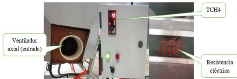
Figure 2. Temperature controller and actuators.
