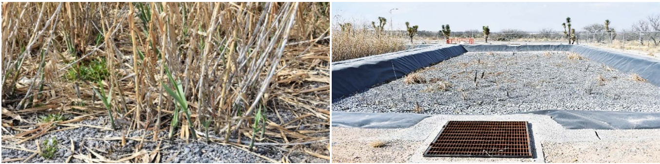
Figure 2. View of the wastewater treatment plant. Vegetation within cell A (left) and complete view of the area (right).
