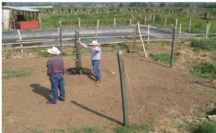
Figure 2. View of the experimental module with separation between poles of 4 m.
